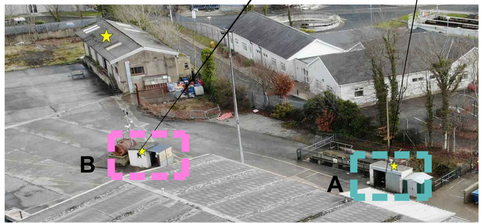
03 IMAGE SHOWING SMALL OUTBUILDINGS TO BE RE-ROOFED. (SEE SITE PLAN ABOVE FOR LOCATION) OUTBUILDINGS SHOWN TO BE RE-ROOFED WITH PROPRIETARY SINGLE PLY MEMBRANE
