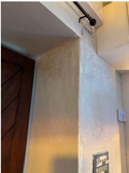
Dampness on wall
