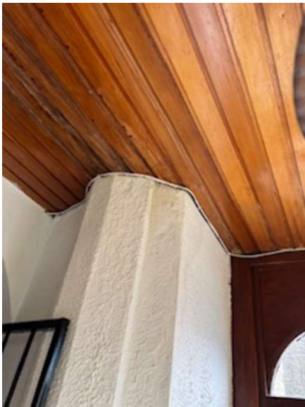
Staining on cladding in porch
