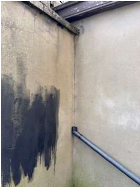
Crack at wall junctions can be filled
