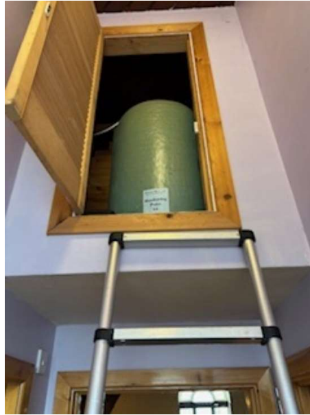
Hot water cylinder.
