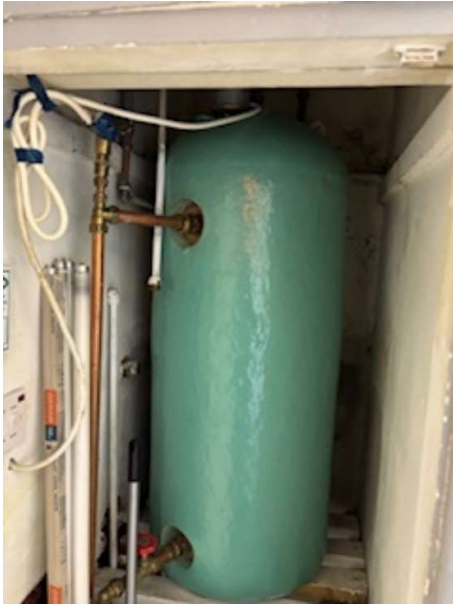
Hot water cylinder
