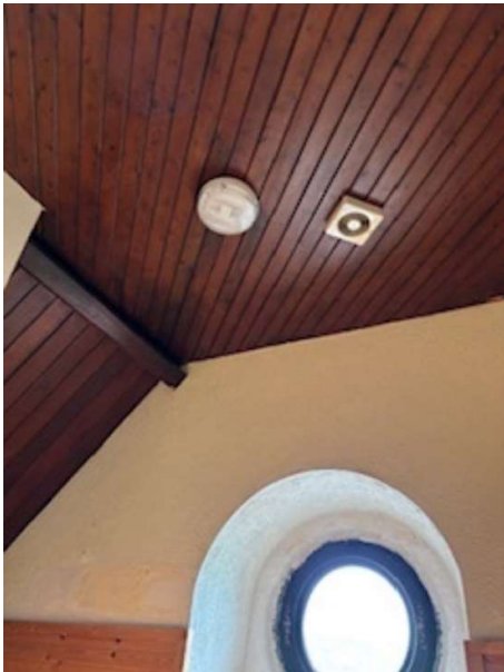
Battery detector Fan in ceiling
