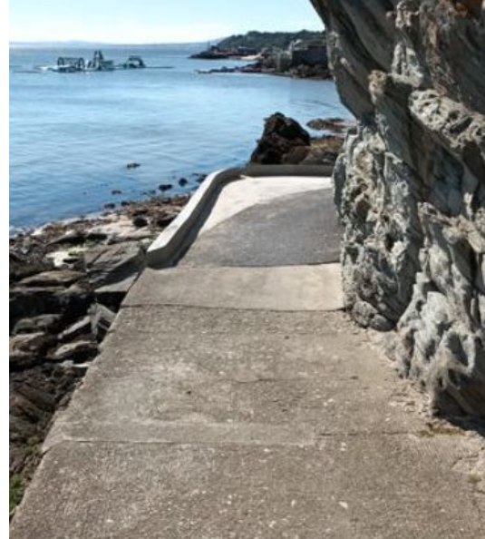
Widened section of path at dangerous bend
